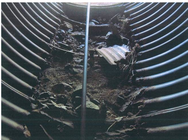
Figure 3.2.4.1 – Culvert invert corroded away
