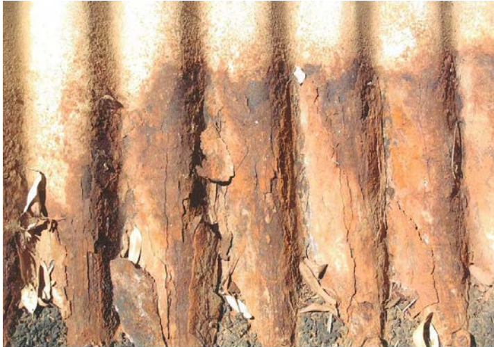
Figure 3.2.3.1(b) – Heavy corrosion
