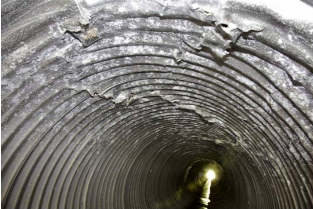
Figure A4 – An aluminium culvert exhibiting local crushing due to corrosion of the upper portion of the culvert
