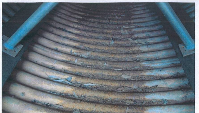
Figure 3.2.2.1 – Culvert showing significant corrosion in invert
