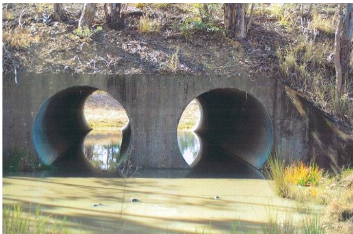
Figure 3.2.1.1 – Standing water in culvert
