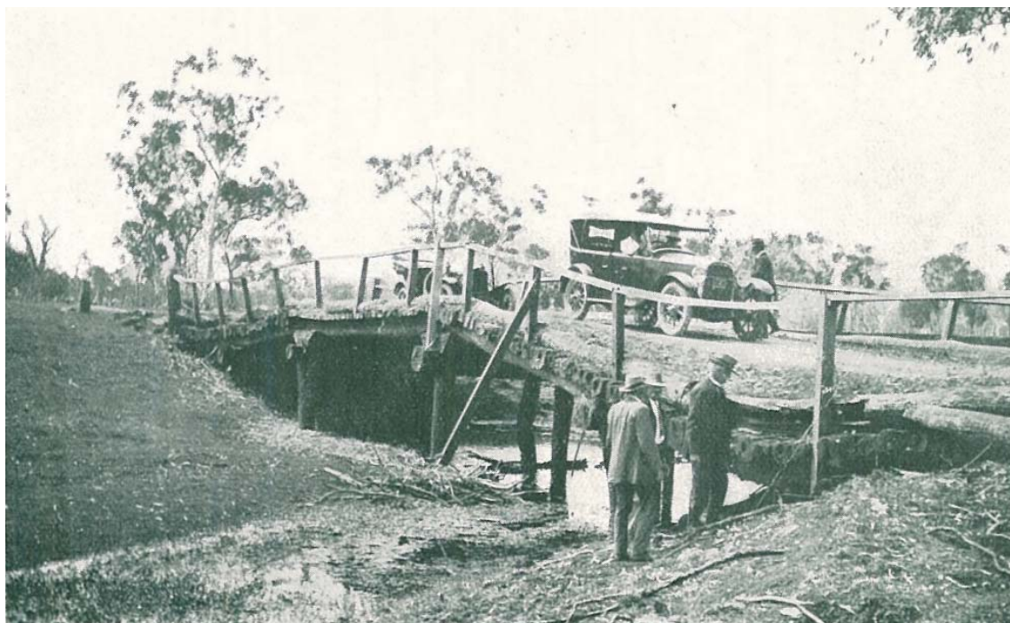
Bridge in a bad state through neglect of maintenance
