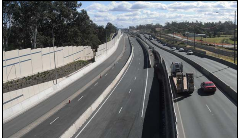
The new permanent pavement through Goodna is nearly ready for the traffic switch next week
