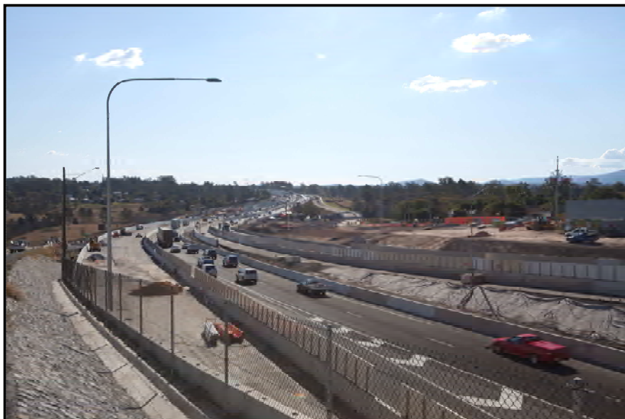
Ipswich bound traffic will be moved slightly south on Saturday night, onto the new permanent alignment through Redbank
