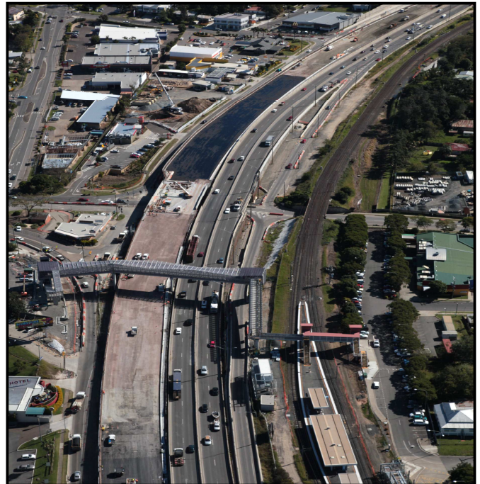
The new Ipswich-bound motorway pavement is close to being completed at Goodna
