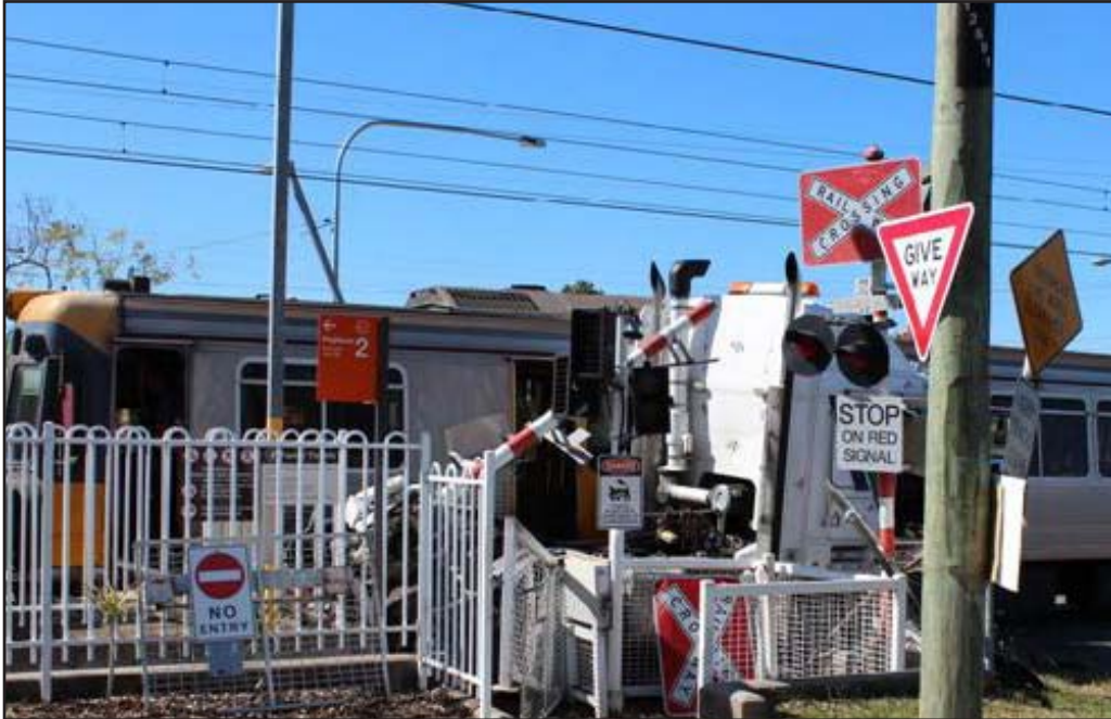
Figure 6: Damage to rail infrastructure
