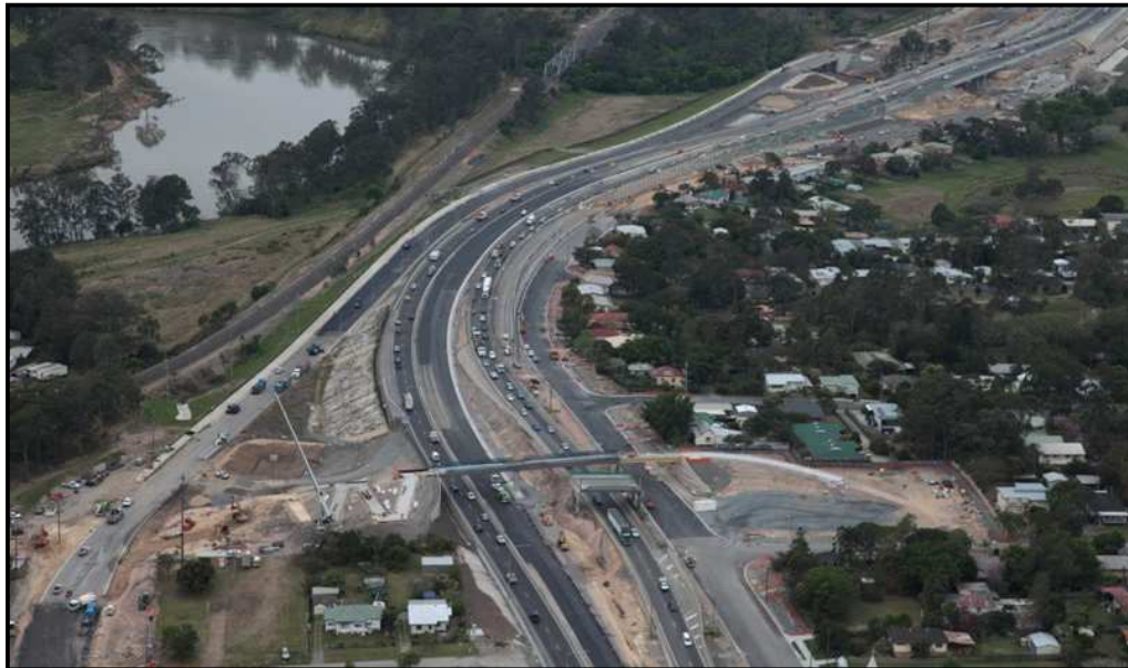
Eastbound view of the works near the Tessman Street pedestrian bridge in Riverview
