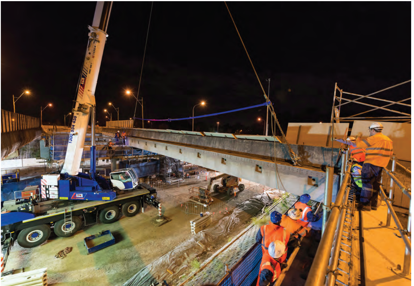
Installation of concrete bridge beams to widen the motorway bridges over Bicentennial Road
