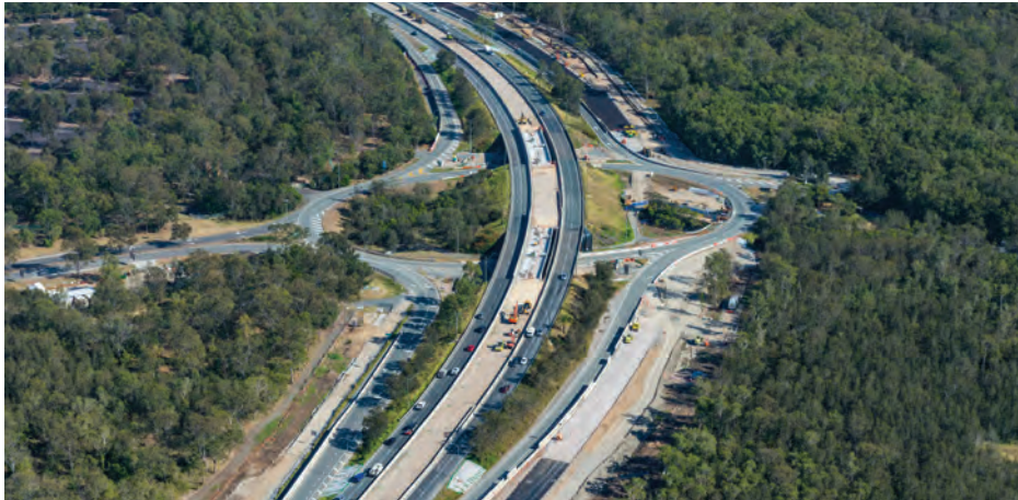
Preparing for the traffic switch at the Bicentennial Road interchange (looking north west)
