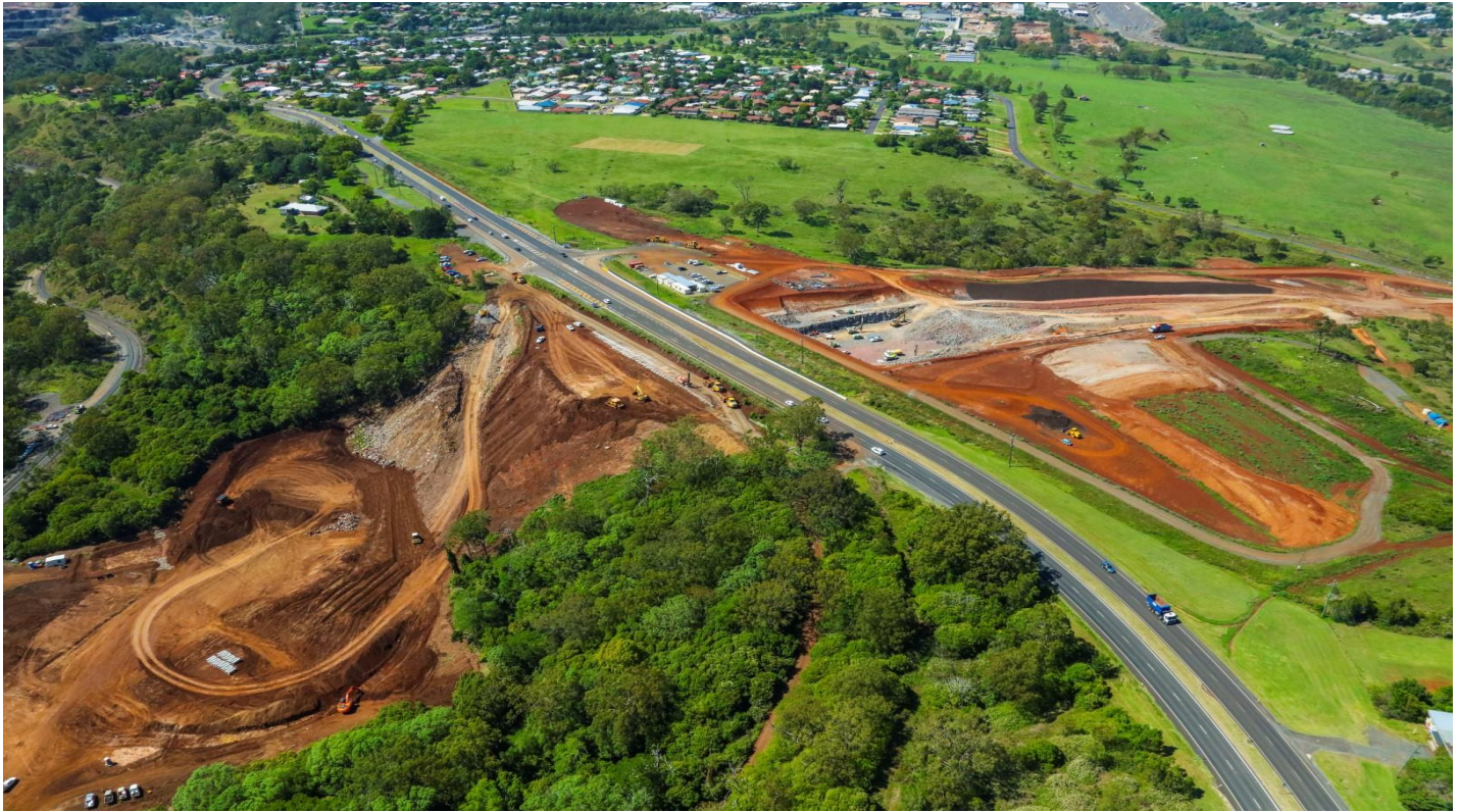
New England Highway, Mount Kynoch with excavation underway for the TSRC cutting, at left, and foundations being laid for twin arch bridges on the New England Highway, at right, where it will pass over the TSRC cutting.
