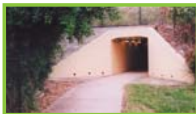
Figure D5-1 Poor visibility and lighting at subways and underpasses can create safety and security issues for pedestrians
