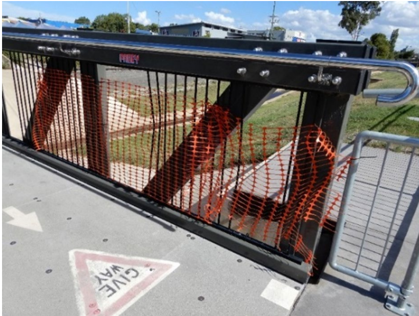
Figure 13.8(b) – Damage to lightweight aluminium balustrade
