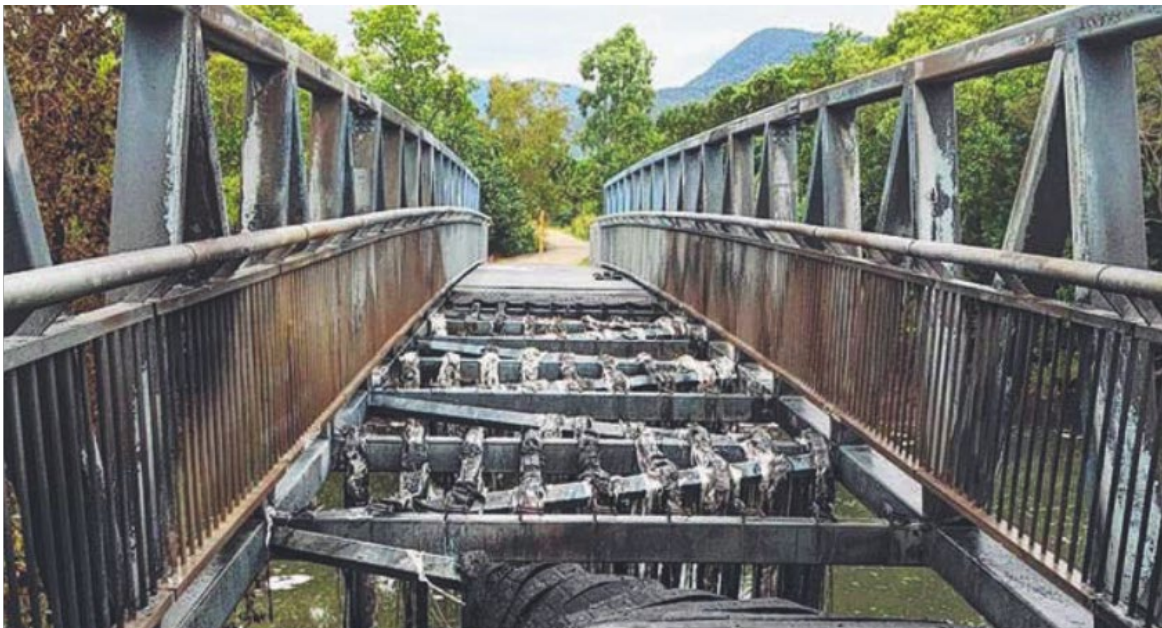
Figure 13.8(a) – Fire damage to recycled plastic deck
