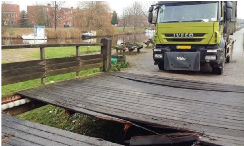
Figure 16 – Bridge deck damage due to inappropriate vehicle access
