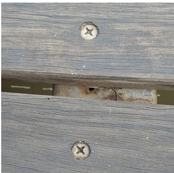
Figure 15.6(c) – Fixing for the timber deck on the bridge over Bulimba Creek (near Ditmas Street)
