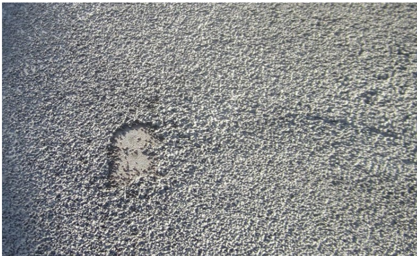
Figure 15.9 – Damage to anti-slip coating on steel deck at Falcon Street
