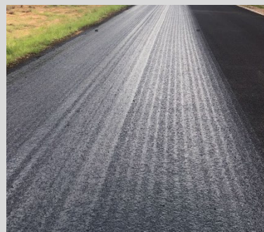
Unacceptable binder uniformity
