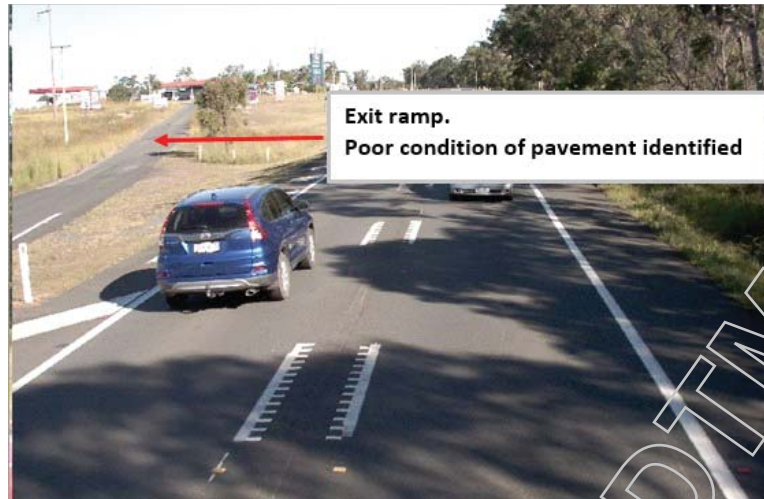
Figure 3 Poor pavement condition
