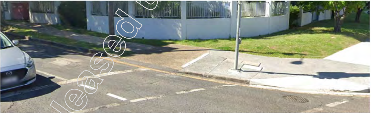
Wellington Road 2 : No gully pit present on upstream side of signalised pedestrian crossing.
