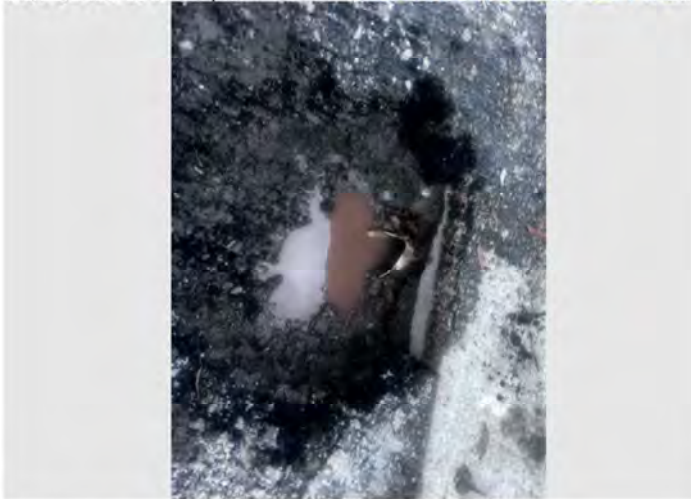
Description End of storm line severed under old footpath
