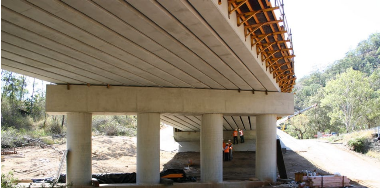
Figure 3.4.1 – Formwork for overhang – prestressed concrete deck unit bridge on small radius curve
