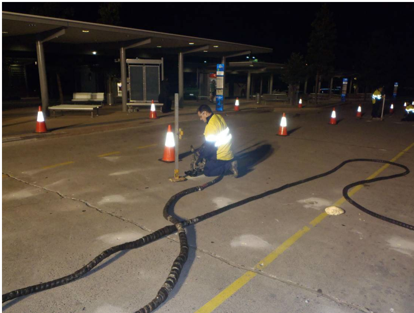
Figure 7(g) – Pressure injecting grout using expanding polyurethane foam – Logan Hyperdome bus station
