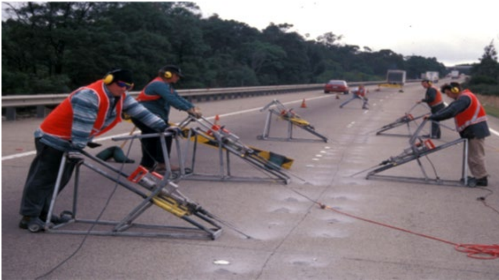
Figure 7(c) – Cross stitching of longitudinal crack
