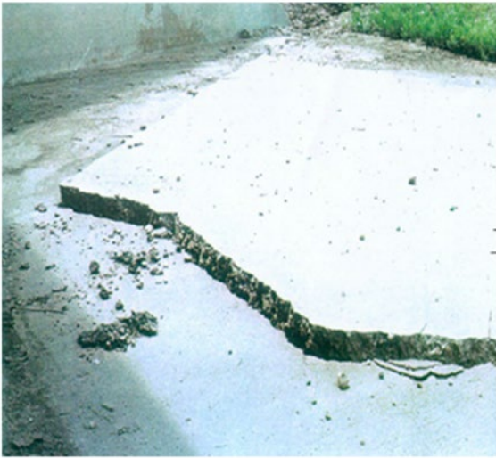
Figure 3.16(b) – Vertical displacement of apron failure
