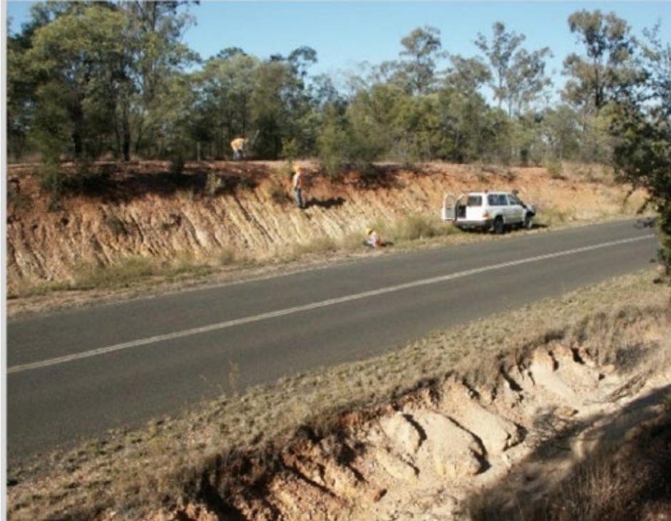
Figure 6B-4 - Example of sodic / dispersive soils in table drains and cut batters
