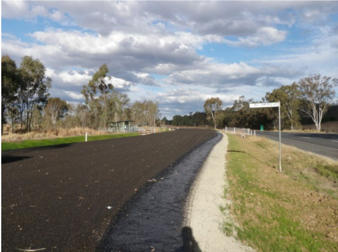
Figure 6B-8 - An economical reseal of an old alignment provides a new rest area with a large capacity
