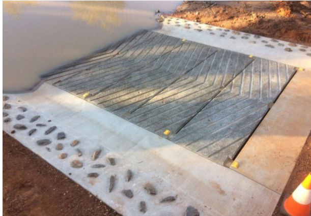
Figure 13.6 – Examples of non-conforming grouted rock shoulder construction
