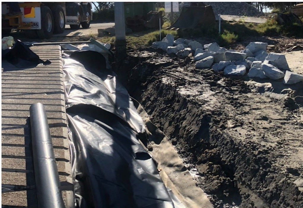
Figure 13.2 – Nonconforming geotextile lining of footing
