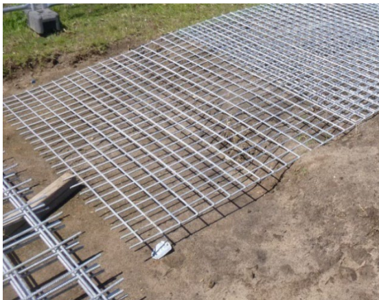
Figure 9.1(b) – Unacceptable storage method
