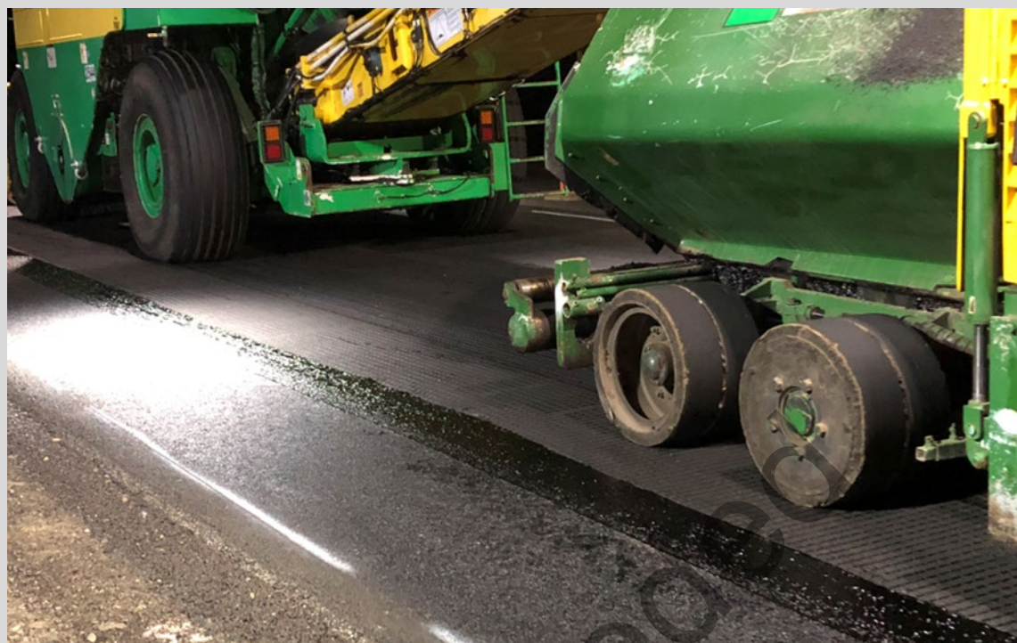
Figure 9.6.3(b) – Minimum bitumen pick-up or wrinkling of the asphalt geosynthetic under the construction plant
