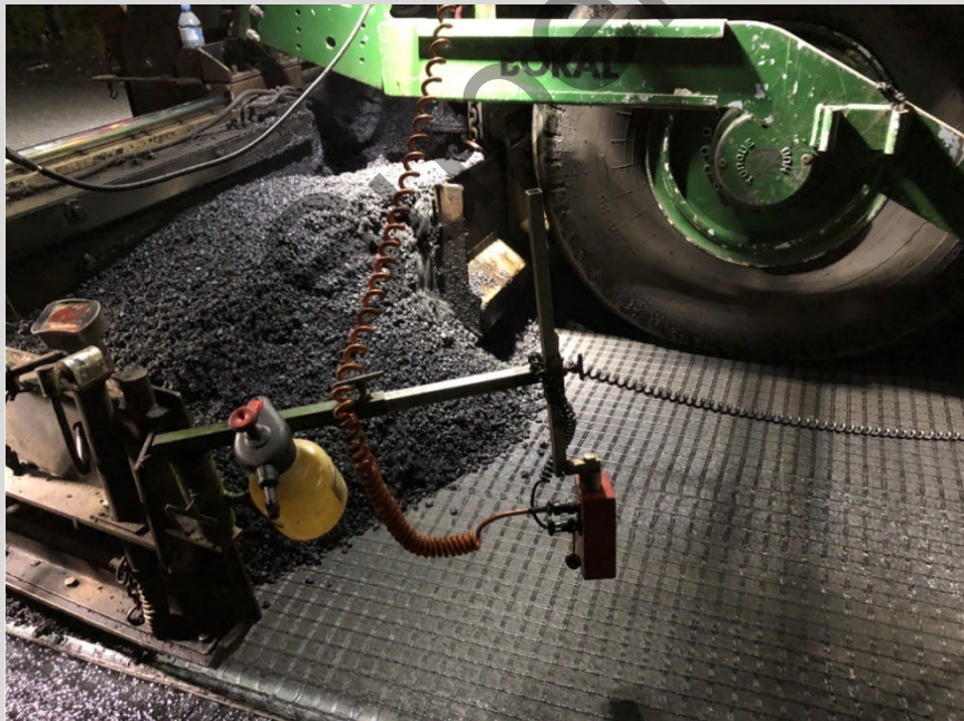
Figure 9.7.1 – Asphalt being paved on asphalt geosynthetic with no bow-waves, wrinkles or folds
