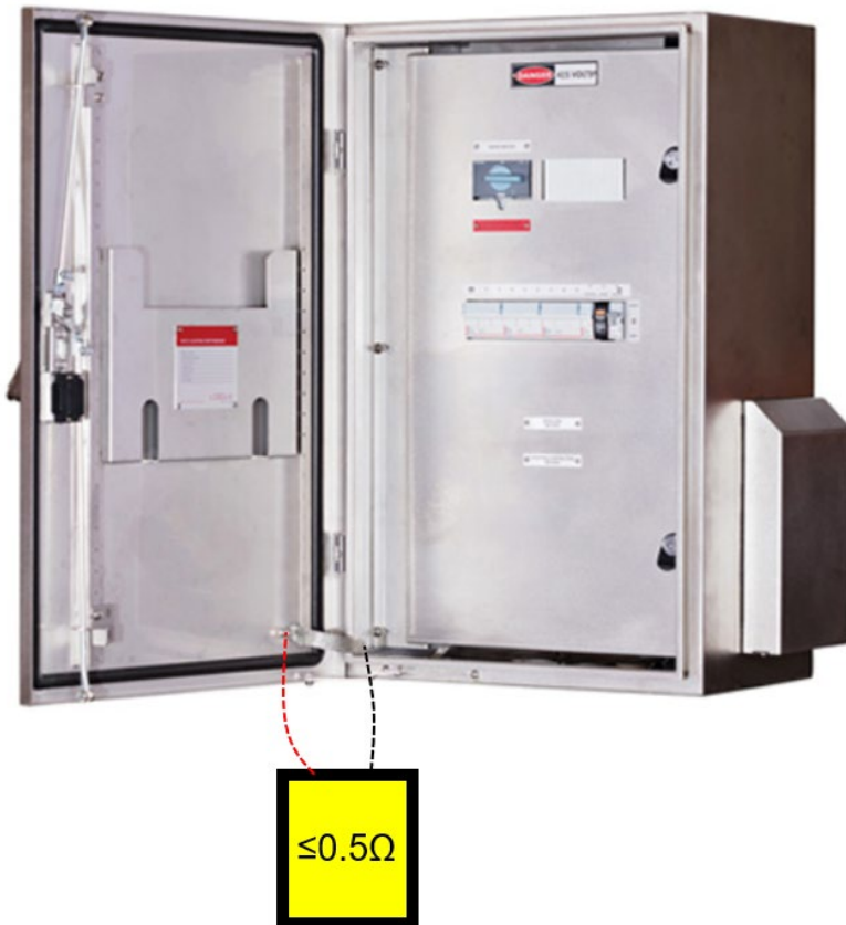
Figure 5.3.2 – Measurement of earth bonding continuity
