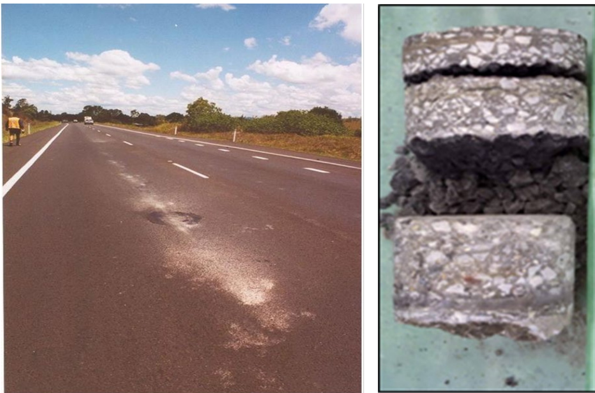
Figure 1 – Example of a stripped asphalt pavement and of a stripped asphalt layer
