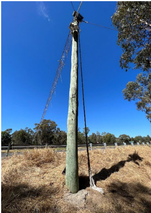
Figure 3.1 – Canopy bridge with degraded rope that requires replacement
