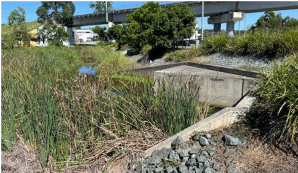
Figure 3.2(b) – Entrance to culvert that is overgrown and requires earthworks and weeding to improve functionality
