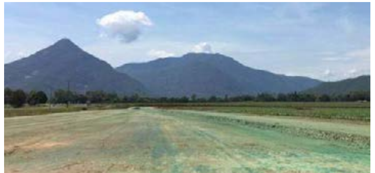
Soil binder securing the materials used to construct the northbound carriageway between Castlereagh Street and Maitland Road.
