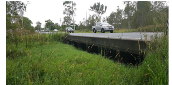
King Johns Creek – existing culverts have low flood immunity
