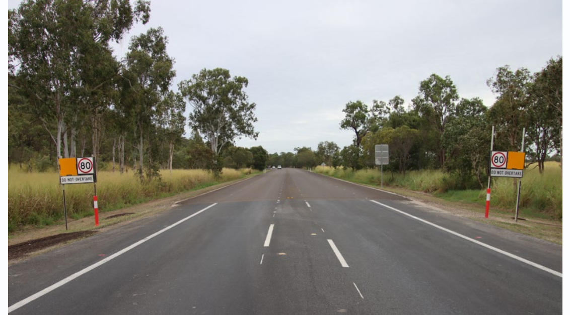
Above: Pavement strengthening undertaken near Hencamp Creek Road, Townsville as part of the Early Start Package. Source: TMR image
