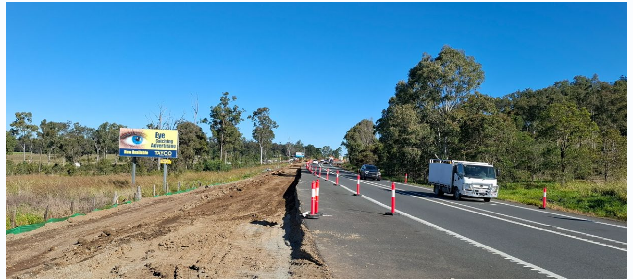
Above: Works are progressing to upgrade the Brooks Road intersection north of Gympie with a channelised right turn facility. Source: TMR image
