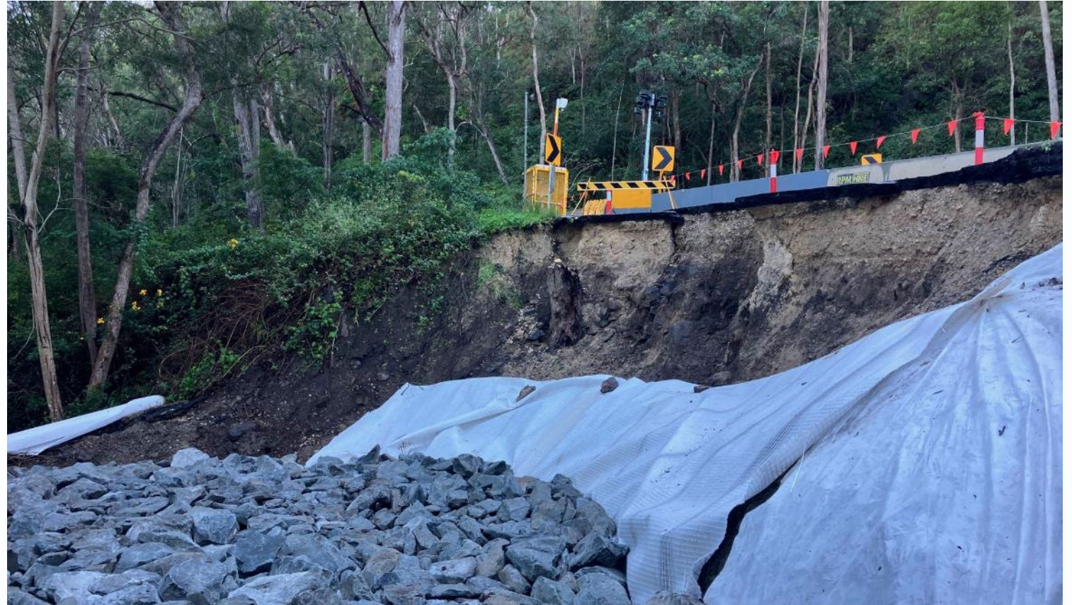
Damaged site associated with Ex-cyclone Alfred
