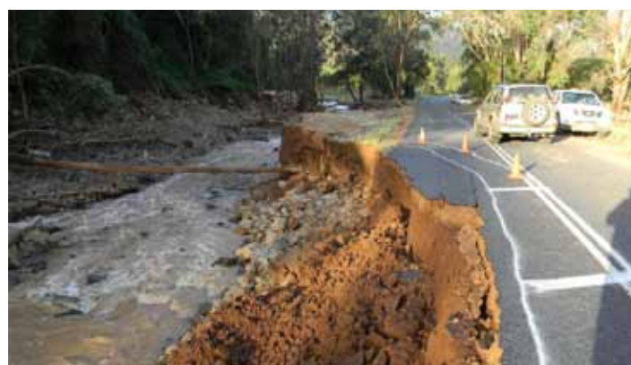
Flood damage on Murphys Creek Road
