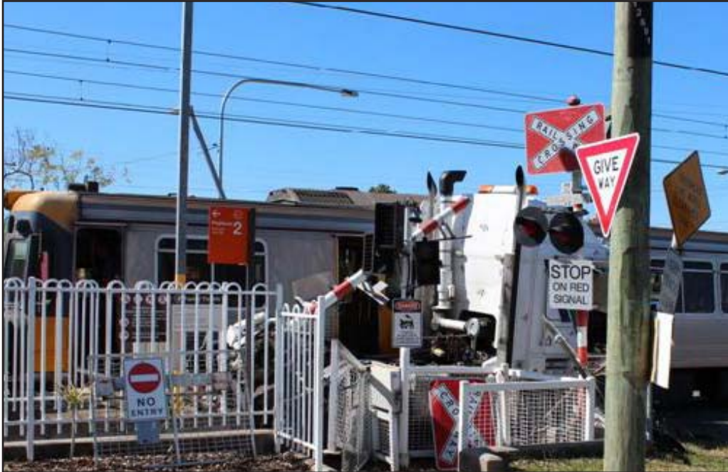
Figure 6: Damage to rail infrastructure
