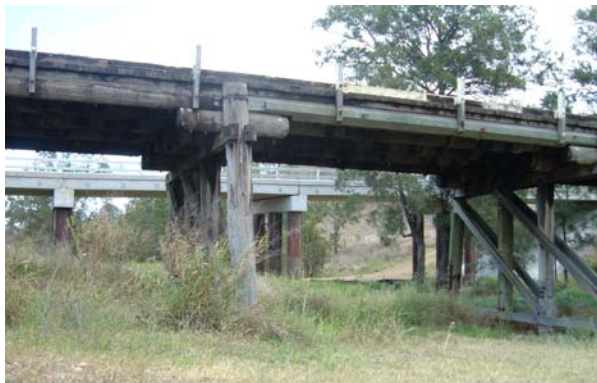
The old timber bridge at Fat Hen Creek, with the new bridge in the background.
