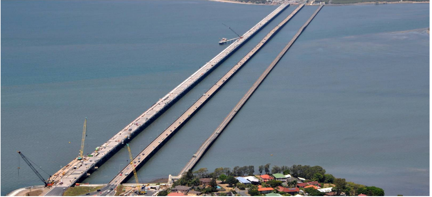
CONSTRUCTION OF THE NEW TED SMOUT MEMORIAL BRIDGE AT CLONTARF IN PROGRESS
