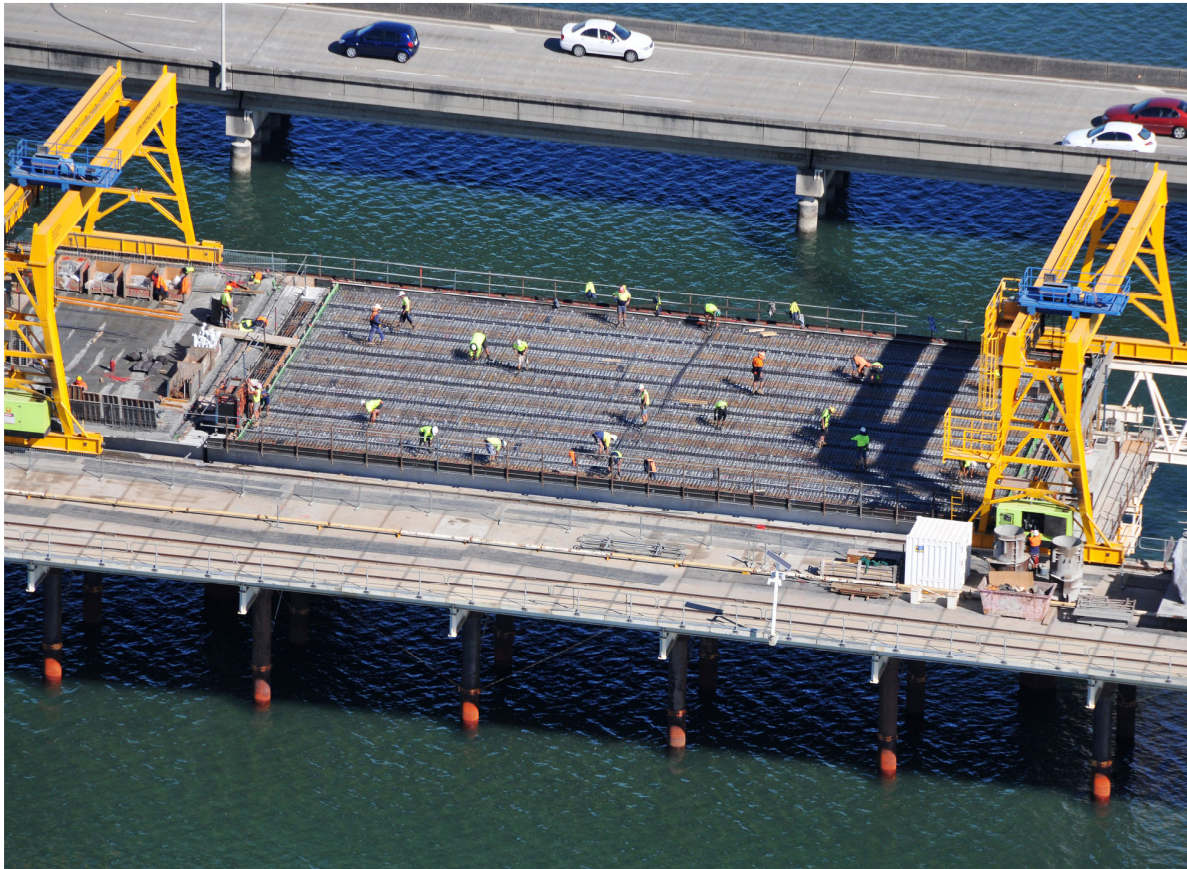
ABOVE: TYING OF STEEL REINFORCEMENT TO ONE OF THE CONCRETE DECKS FOR THE NEW TED SMOUT MEMORIAL BRIDGE.
