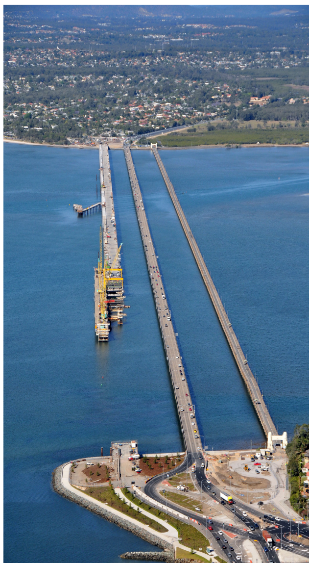
ABOVE: CONSTRUCTION OF THE NEW TED SMOUT MEMORIAL BRIDGE ADVANCES ACROSS BRAMBLE BAY TOWARDS CLONTARF POINT.
