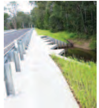
After guard rail
