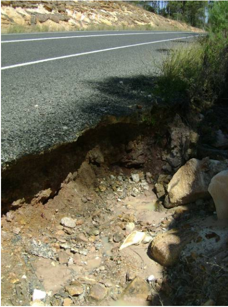
Figure 6B-5 - Undermining of road asset by erosion of sodic / dispersive soils
