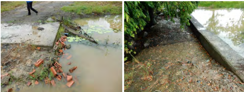
Plate 3: Collapsed road culvert downstream (left) and concrete weir located downstream (right) of the crossing point on Traveston Creek
